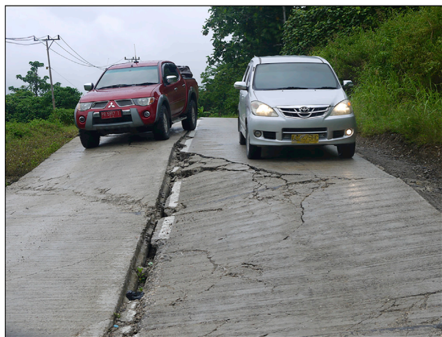
Figure 3. Potholes and slumping in tropical roads.
